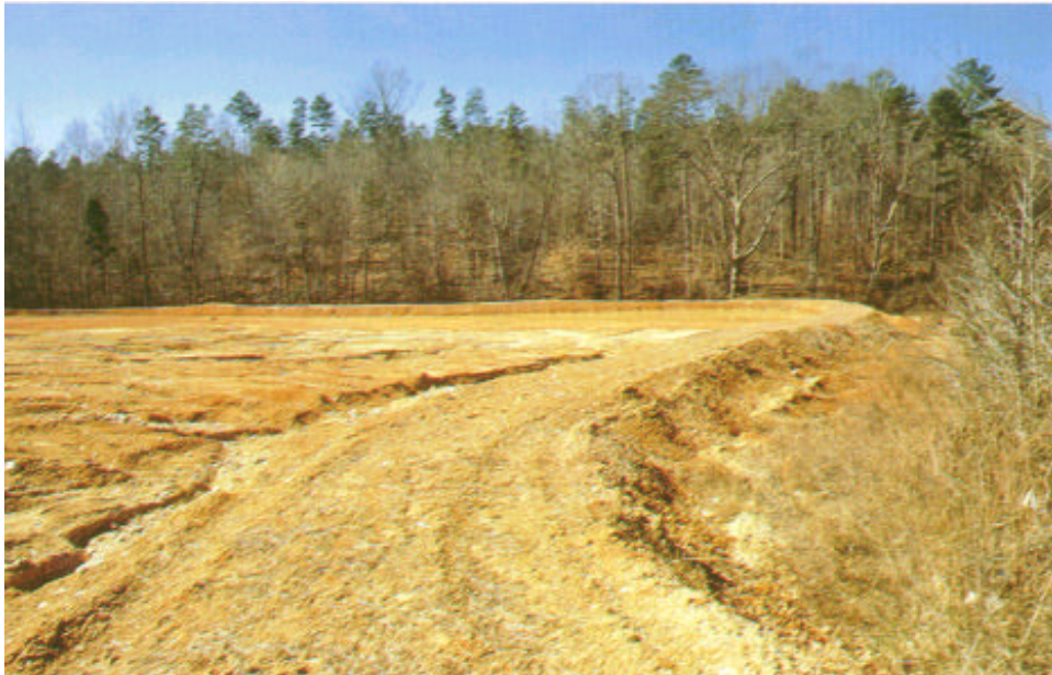
Perimeter protection diversion protects work areas and prevents sediment from leaving the site.
